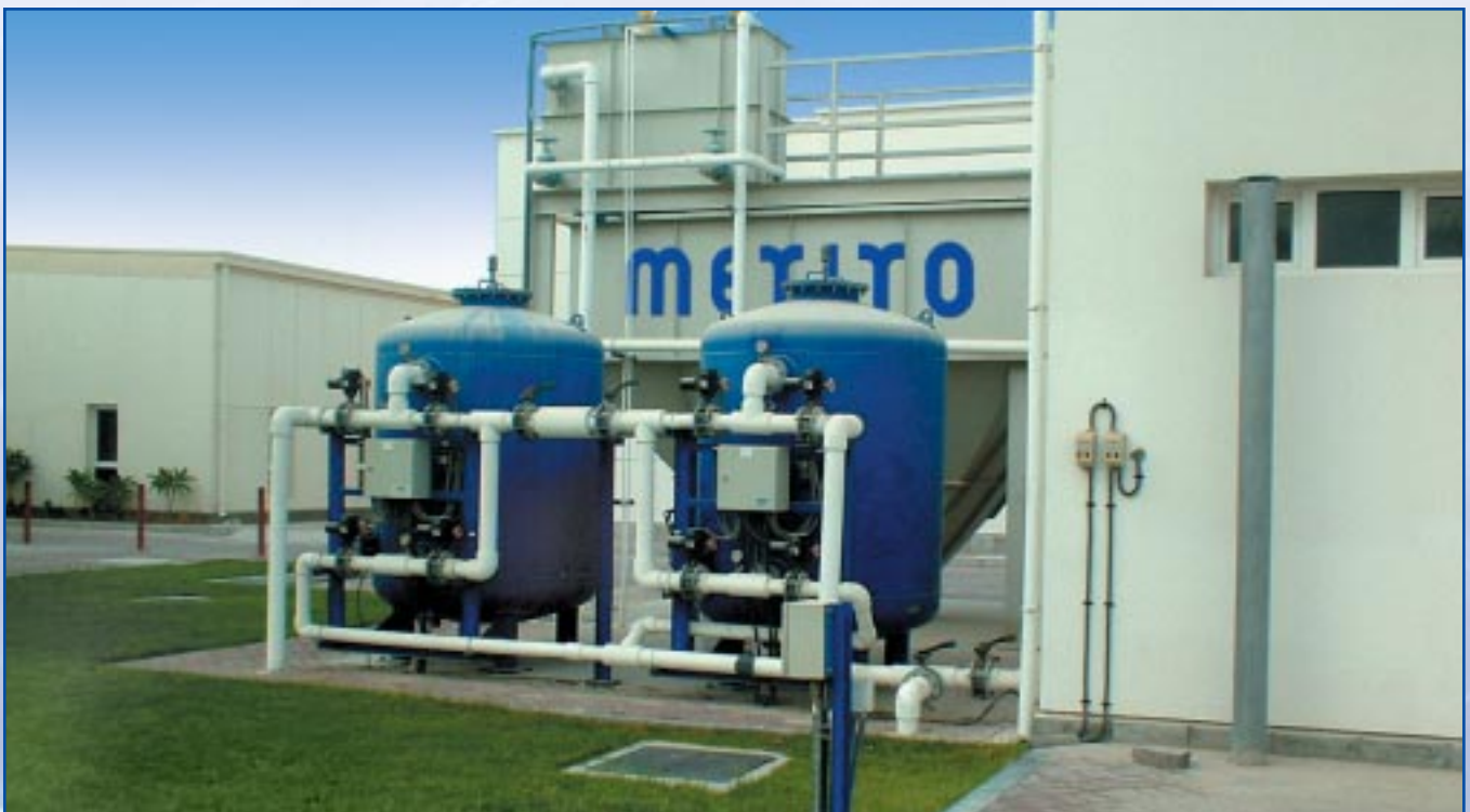
METITO Sanicycler® System Installed at a Housing Compound
