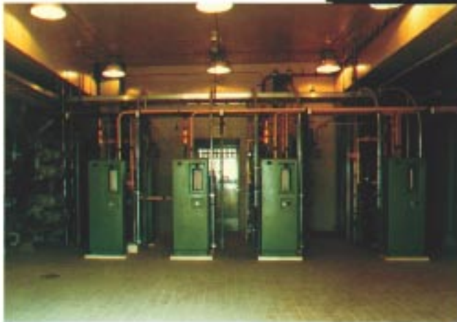
Chlorination plant installed in the U.A.E.
