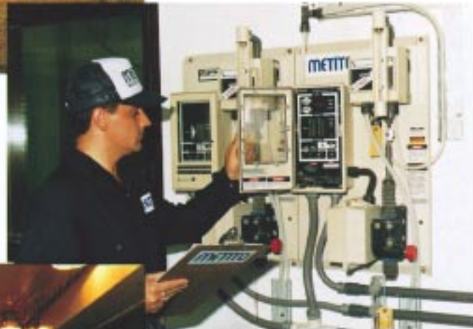
Chlorination control and measurement facilities
