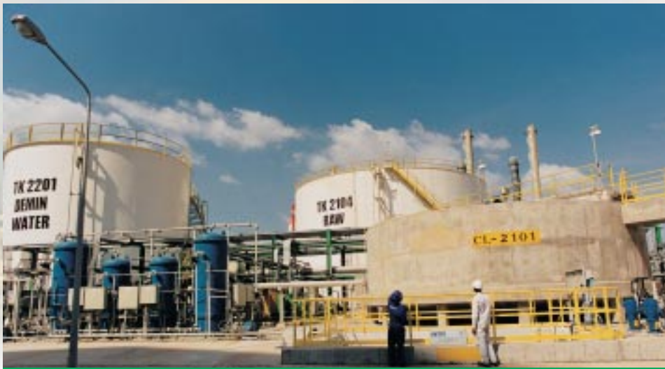
FULLY AUTOMATIC DEMINERALIZATION & WATER PRE TREATMENT PLANTS
