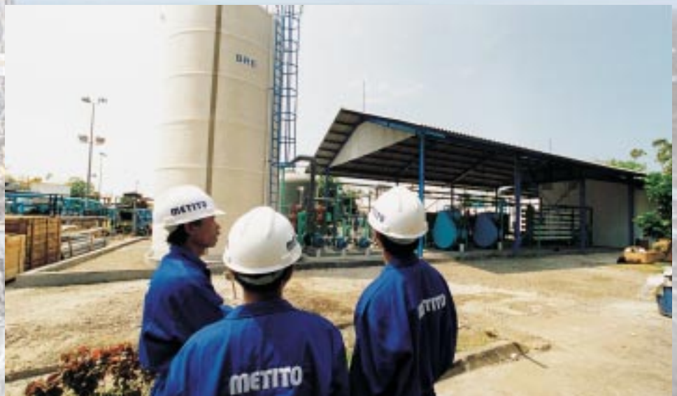
OVERALL VIEW OF THE DESALINATION PLANT
