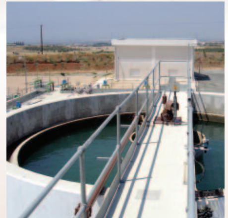
A VIEW OF THE SLUDGE THICKENER
