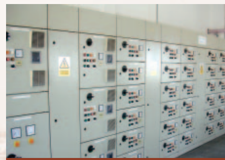
THE MOTOR CONTROL CENTER
