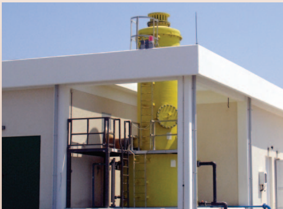
THE CHLORINE NEUTRALIZATION TOWER
