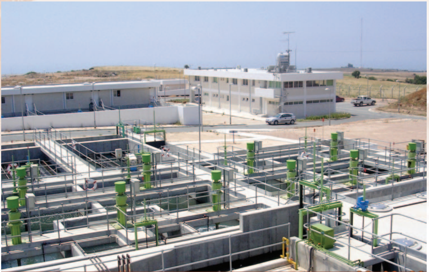
A VIEW OF THE FLOCCULATION CHAMBERS AND LAMELLA CLARIFICATION UNITS
