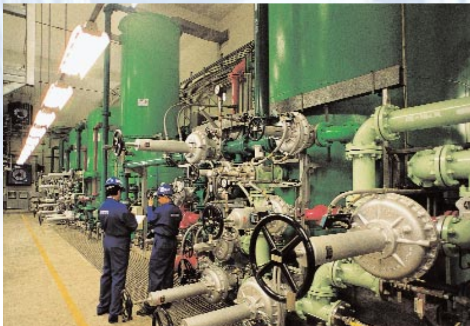
Nest of pneumatically operated automatic valves
