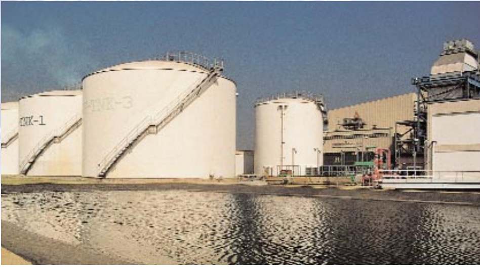
Demineralization plant water storage tanks
