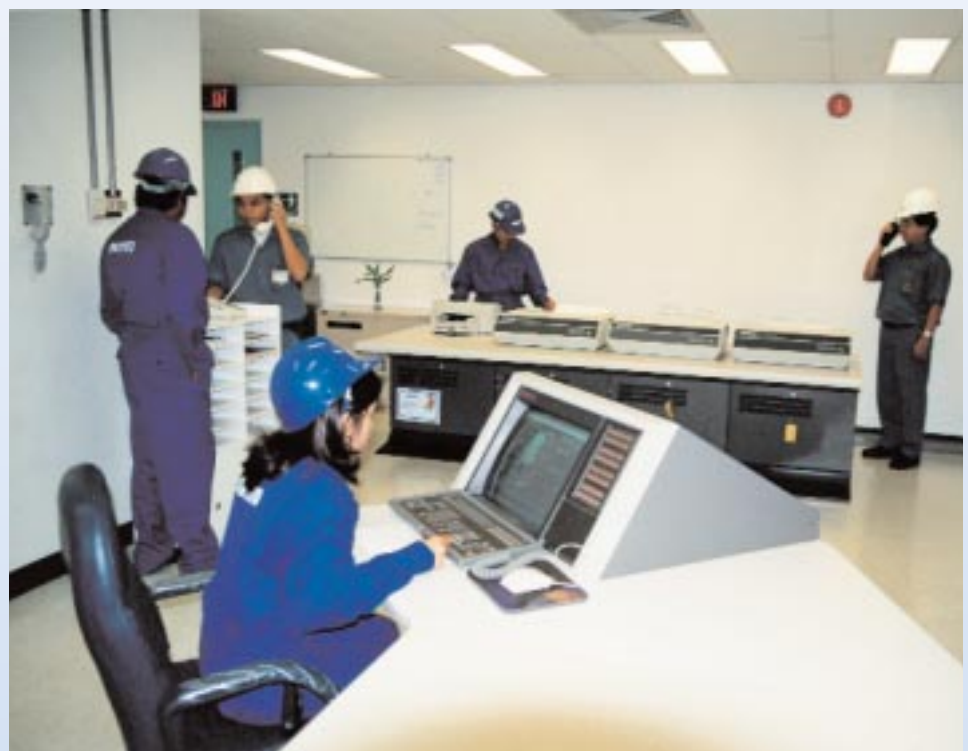
Distributed control & information system room
