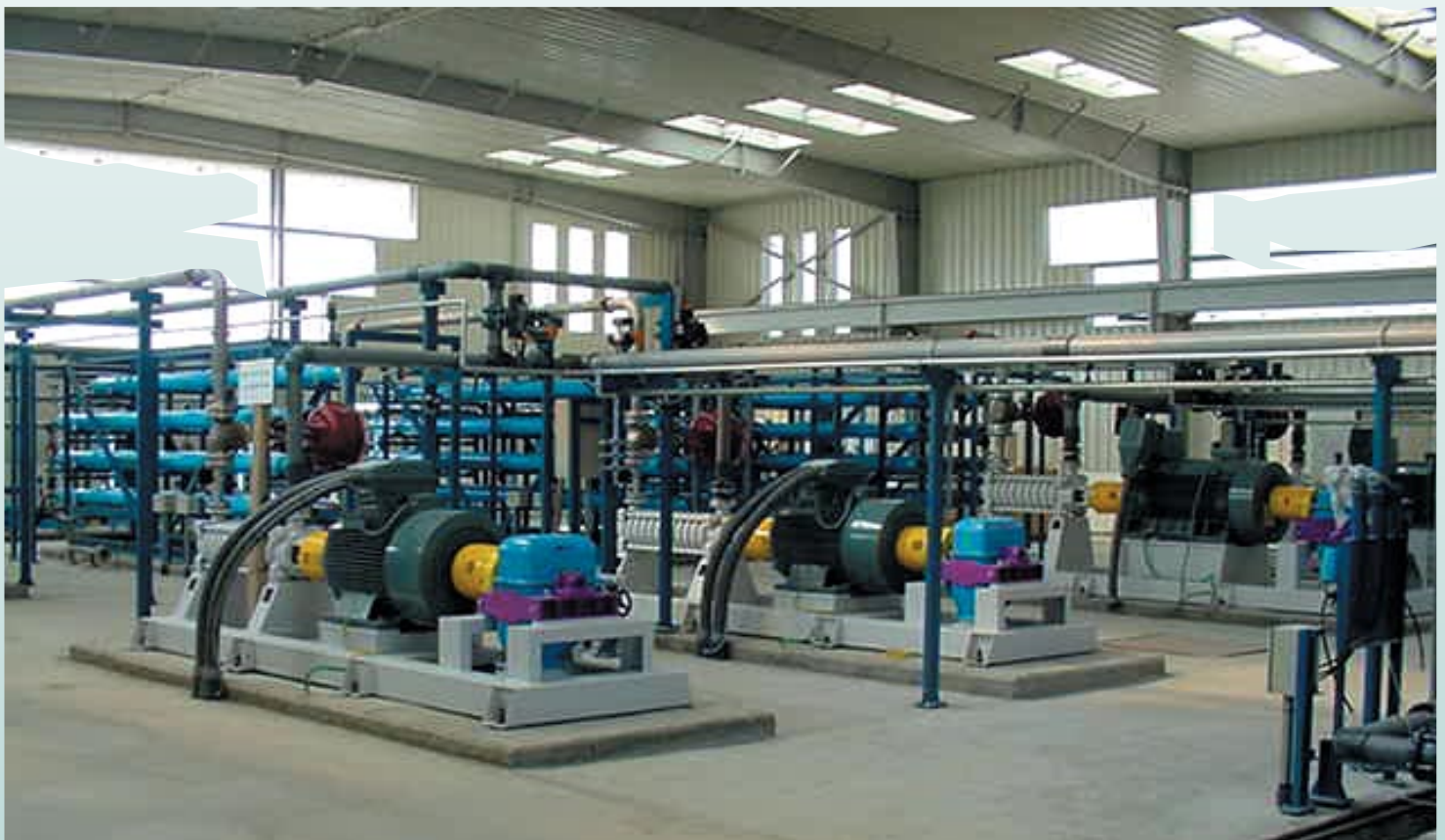
AN OVERVIEW OF THE SEAWATER REVERSE OSMOSIS PLANT ROOM
