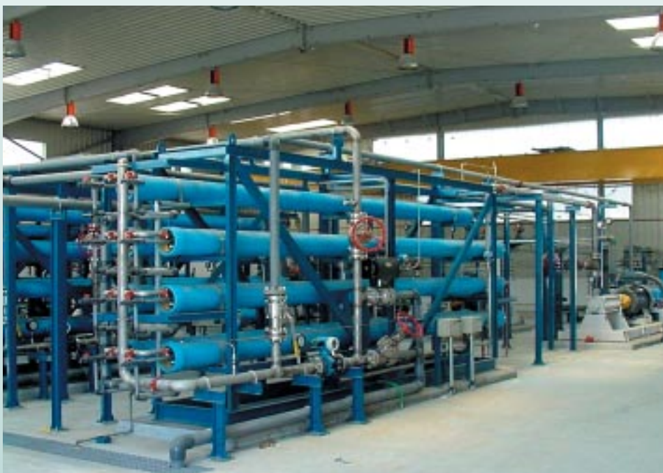
A VIEW OF A REVERSE OSMOSIS STREAM
