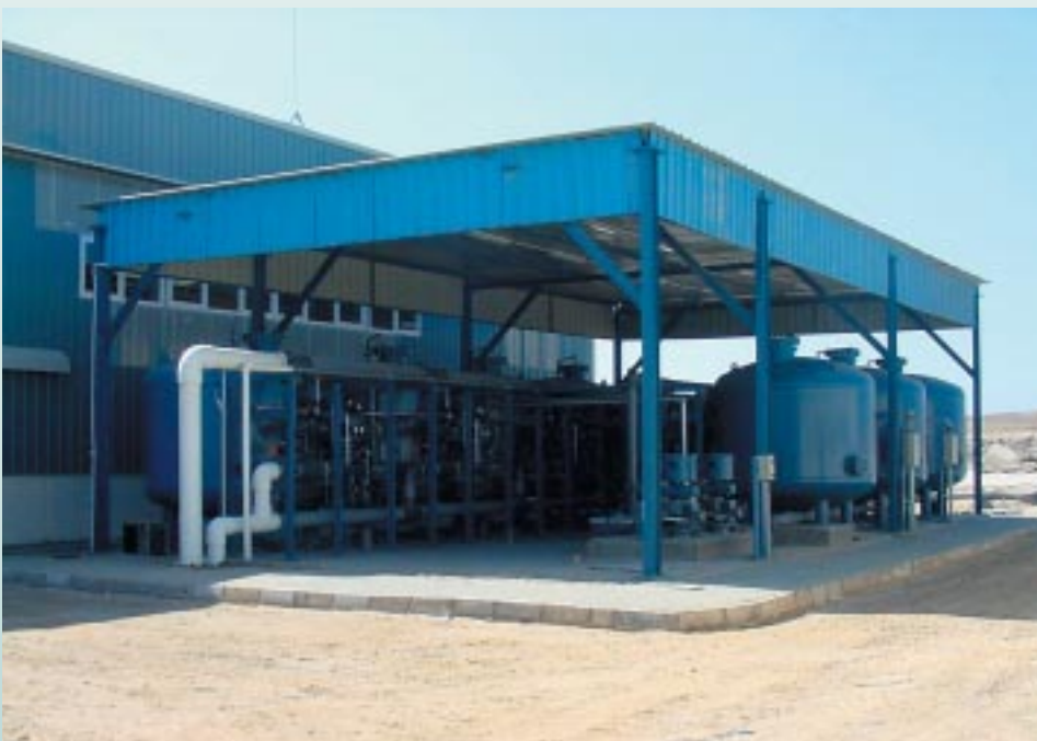
THE MULTI-MEDIA FILTRATION SYSTEM
